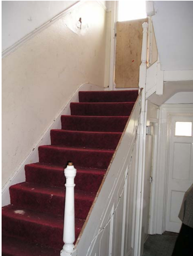
Hallway showing extensive damage to staircase
