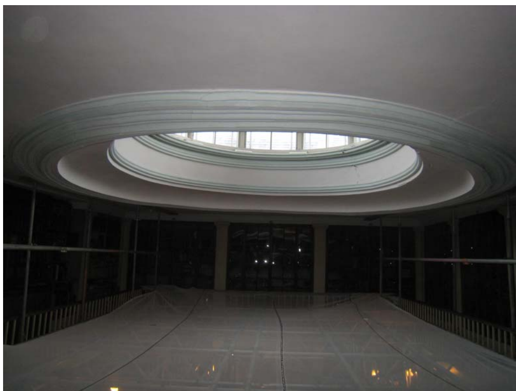
The dome is dropping into the library. The structure is currently supported by scaffolding, with netting to catch any falling debris.
